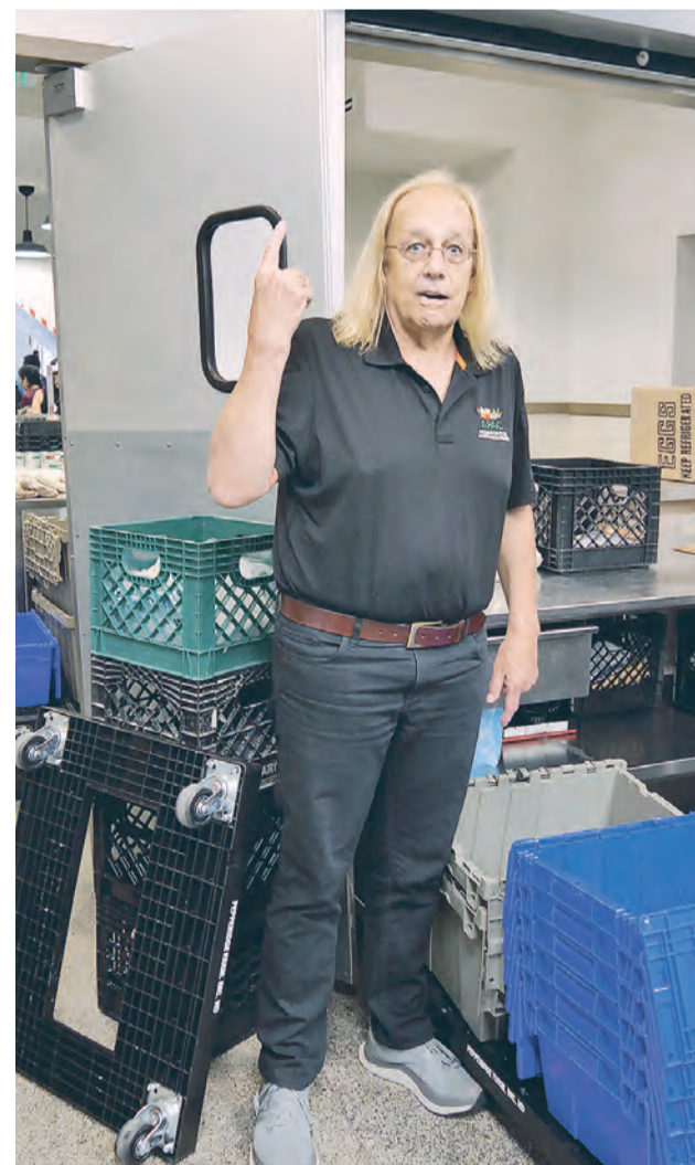
Charles Meng shows his early office at AFAC where water dripped on his head from a leak in the ceiling.
